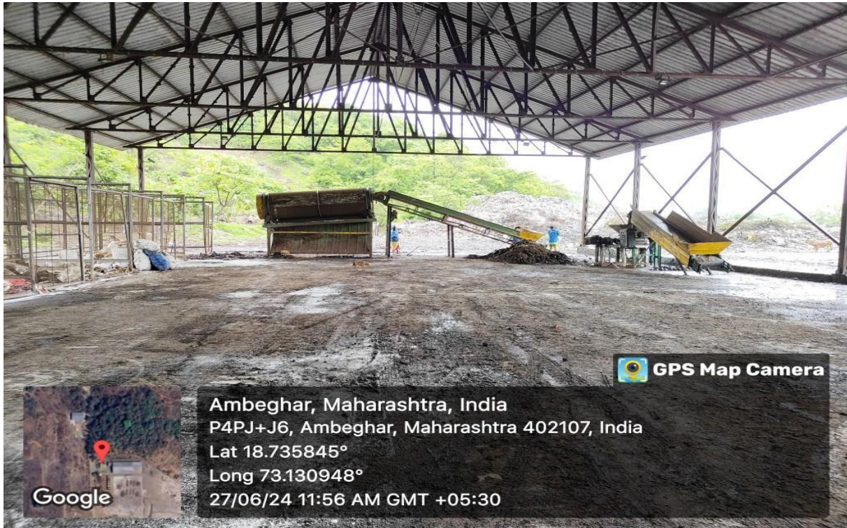
Photograph-5: Screening machine of organic waste convertor installed for processing of wet waste.
