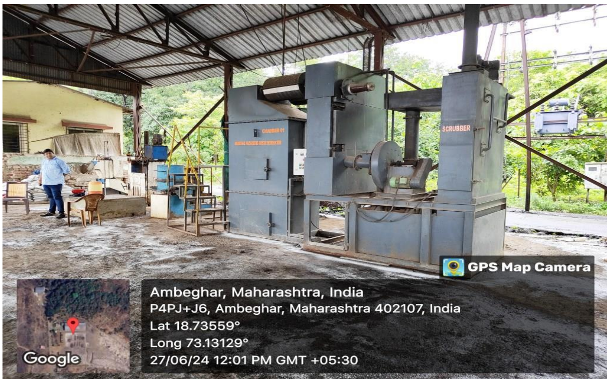
Photograph-6: Domestic hazardous waste incinerator installed for processing of domestic hazardous waste.
