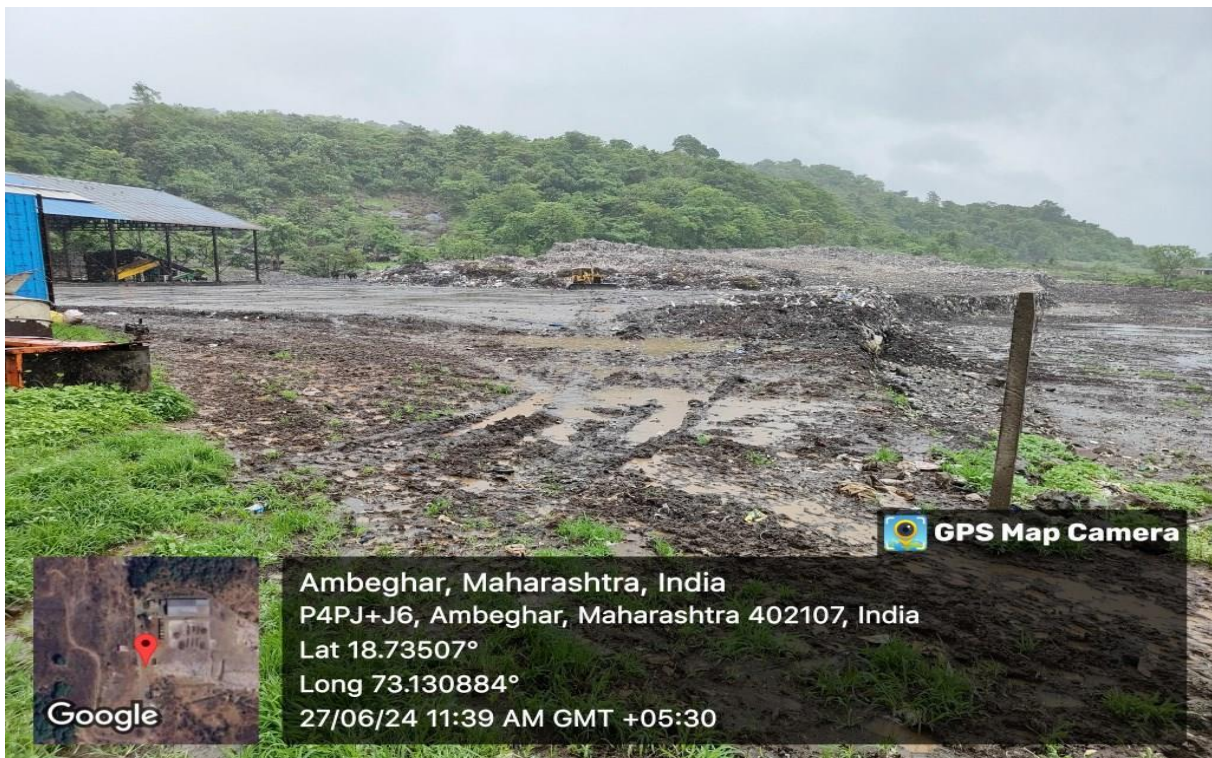
Photograph-2: Legacy waste stockpiled within the Survey no. 156 and solid waste processing facility without fencing around the boundary to prevent spillages of solid waste and entry of unauthorized persons & stray animals.
