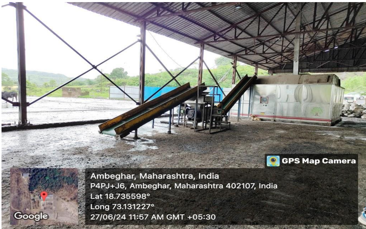
Photograph-4: Organic waste converter installed for processing of wet waste.
