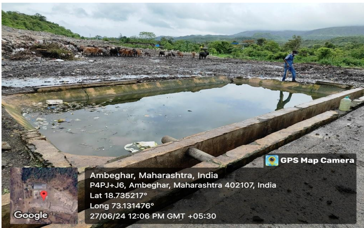
Photograph-8: Lined leachate collection pit for management of leachate.
